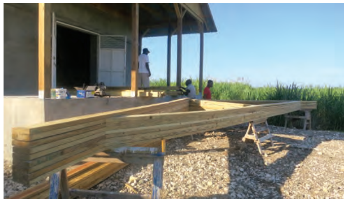
We source construction supplies in Haiti and then assemble roof trusses at our warehouse.
