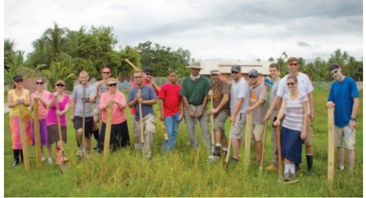
Above: The team from Second Houston broke ground on the Trade School campus—located on our Signeau Elementary School property—on the main highway in Haiti.
