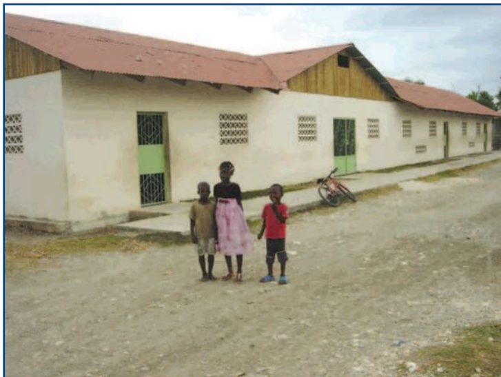
The New Missions Ti Rivierre elementary school has received several repairs and updates such as new doors and wood paneling. Painting the building is next on the list.
