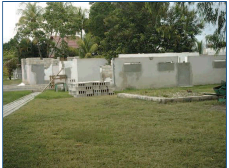
The first building at New Missions, commonly called the U-shape building, was home to our office, clinic, and missionary housing. This building is receiving a new roof and upgrades.
