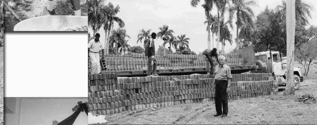
A businessman from our church in Sosua donated a truckload of cement blocks for the construction of our buildings. When another businessman heard of it, he donated a hundred sacks of cement. God has promised to provide.
