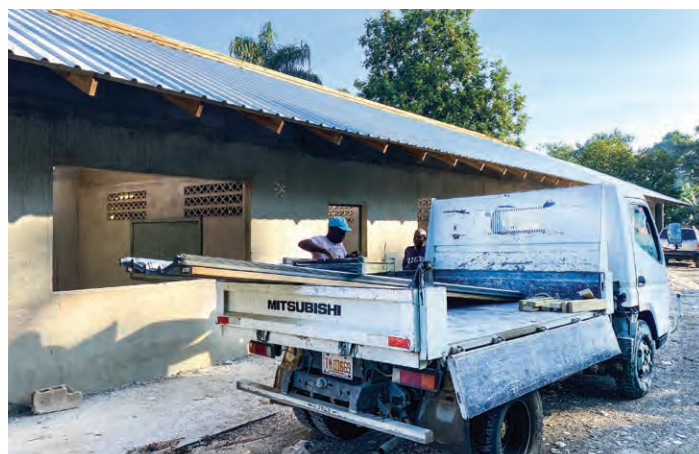
Roofing supplies are now available. Pictured here, the roof in Lassale is almost finished.
