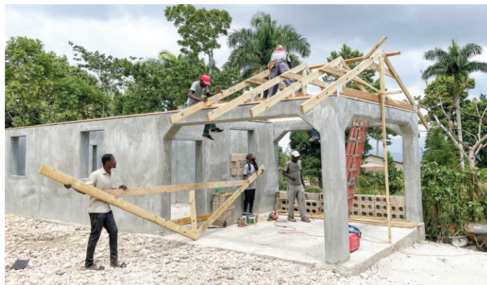
Trusses, which will be covered with metal roofing, are going up on new Tom Gateau kitchen.
